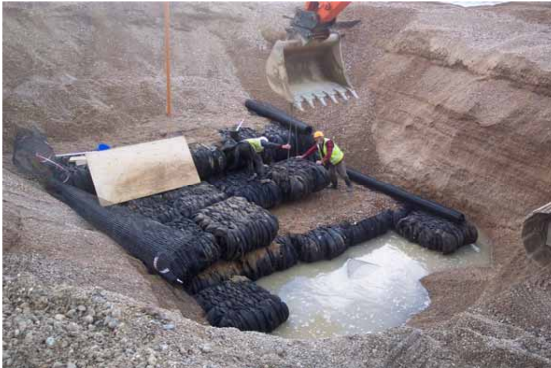
Figure 5.29 Installation of bales in the beach at Pevensey Bay in East Sussex (courtesy PCDL)
