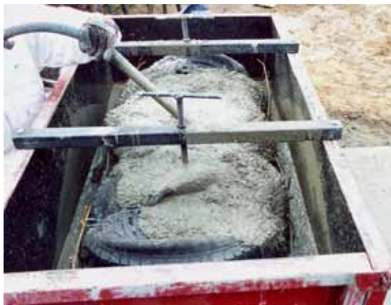
Figure 5.40 Concrete being poured around tyre bale into block cast (courtesy Northern Tyre recycling)
