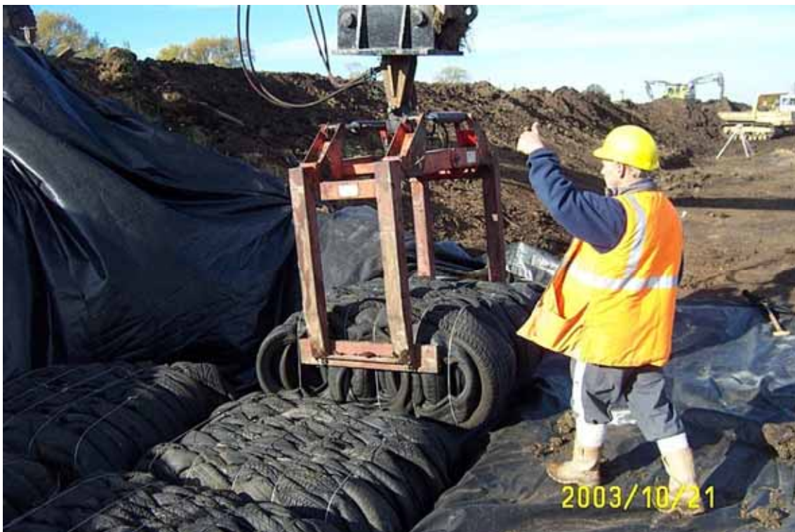
Figure 4.7 Placement of tyre bale into structure using a pallet grab attachment (courtesy Environment Agency)
